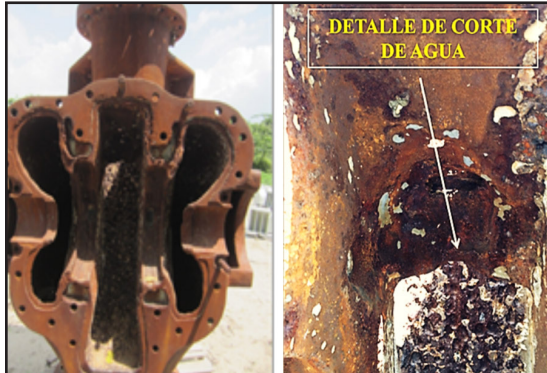
Pump body as inspected
